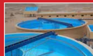
Water Treatment Plant Saudi Arabia
